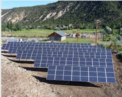
Holy Cross Energy community solar array, operated by the Clean Energy Collective
