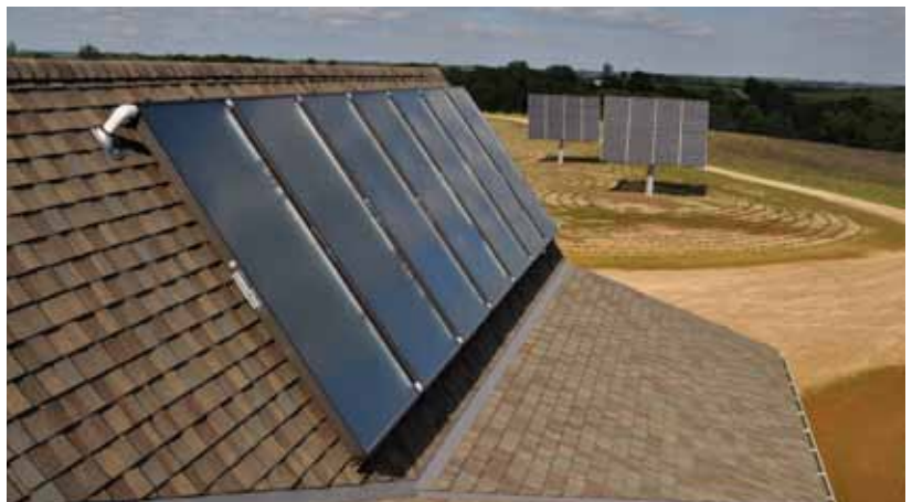
Residential solar hot water with ground-mounted PV in Viola, Wisconsin
