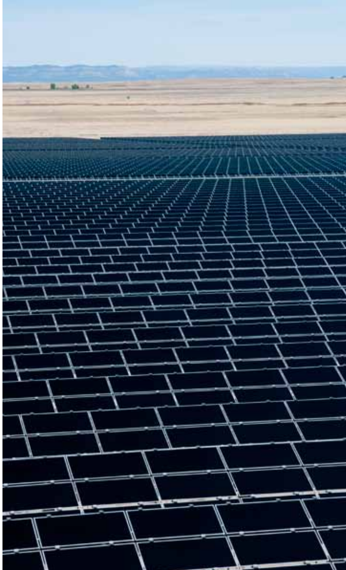
30-MW installation in Cimaron, New Mexico
