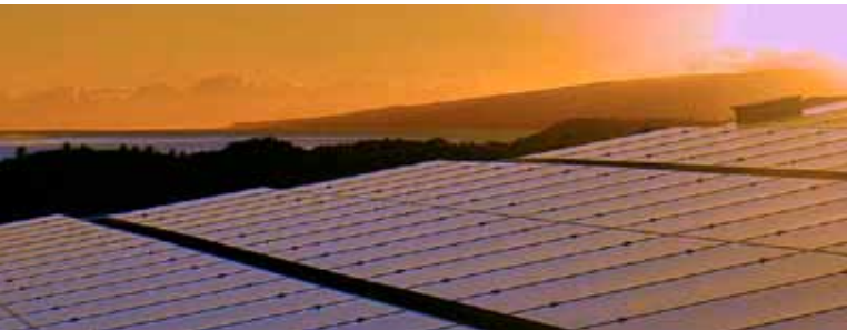
Photovoltaic installation on Molokai General Hospital, Hawaii Photo by Shanti Berg, ProVision Solar
