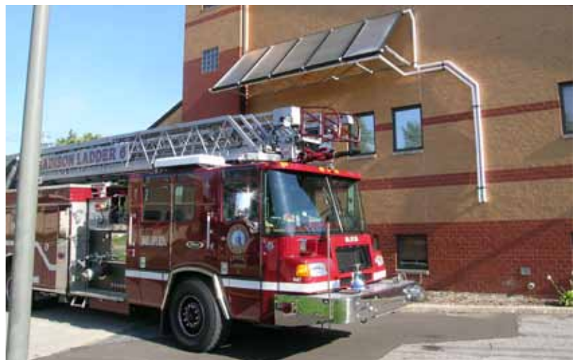
Solar hot water installation at Fire Station in Madison, Wisconsin
