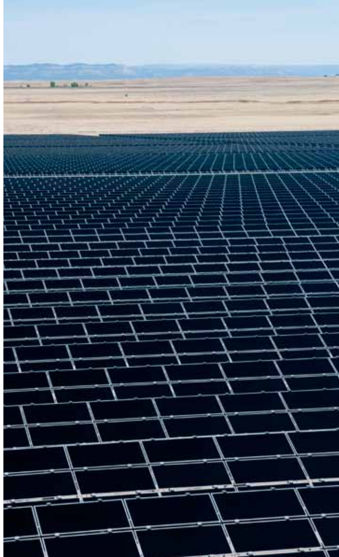
30-MW installation in Cimaron, New Mexico
