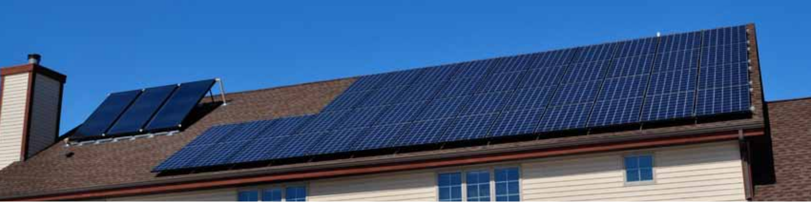
Residence with photovoltaics and solar hot water in Fitchburg, Wisconsin
