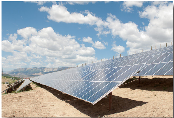
Community solar installation in Rifle, CO
