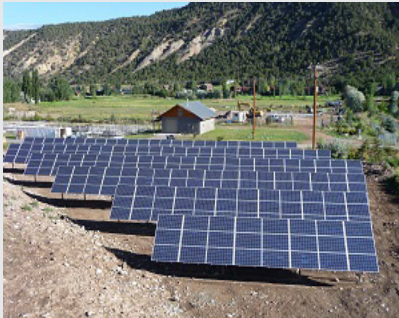
Holy Cross Energy community solar array, operated by the Clean Energy Collective
