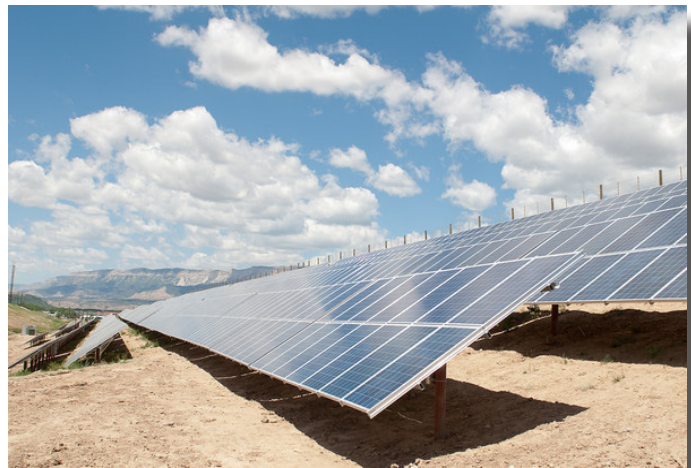
Community solar installation in Rifle, CO .
