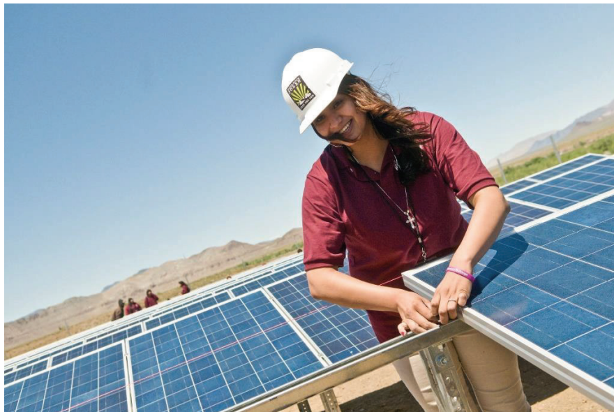
A 135 kW system at Pyramid Lake Paiute Tribe High School in Nixon, NV. (Photo: Black Rock Solar)
