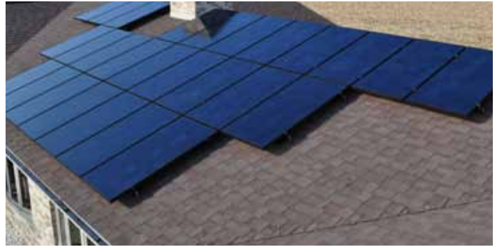
Residential solar installation in Columbus, Wisconsin
