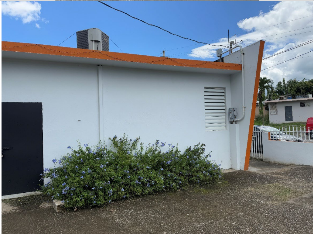
Proposed area for Designer consideration for DER and BESS installation
